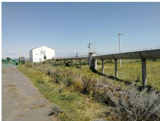
Figure 22: Wastewater Treatment Plant in Artsvakar District of Gavar Town (2018)
