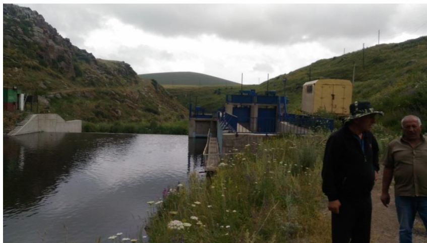
Water Abstraction Structure
